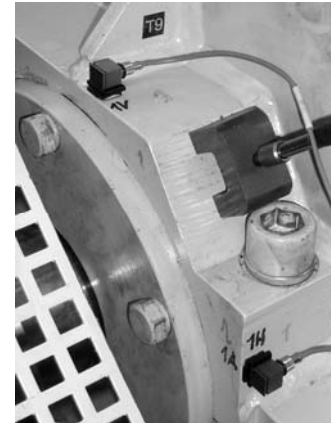
Fig. 4 Accelerometers placing on the gearbox housing
